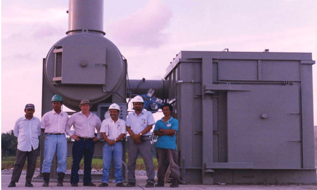
BOS system installed at Mobil Oil refinery in Indonesia
