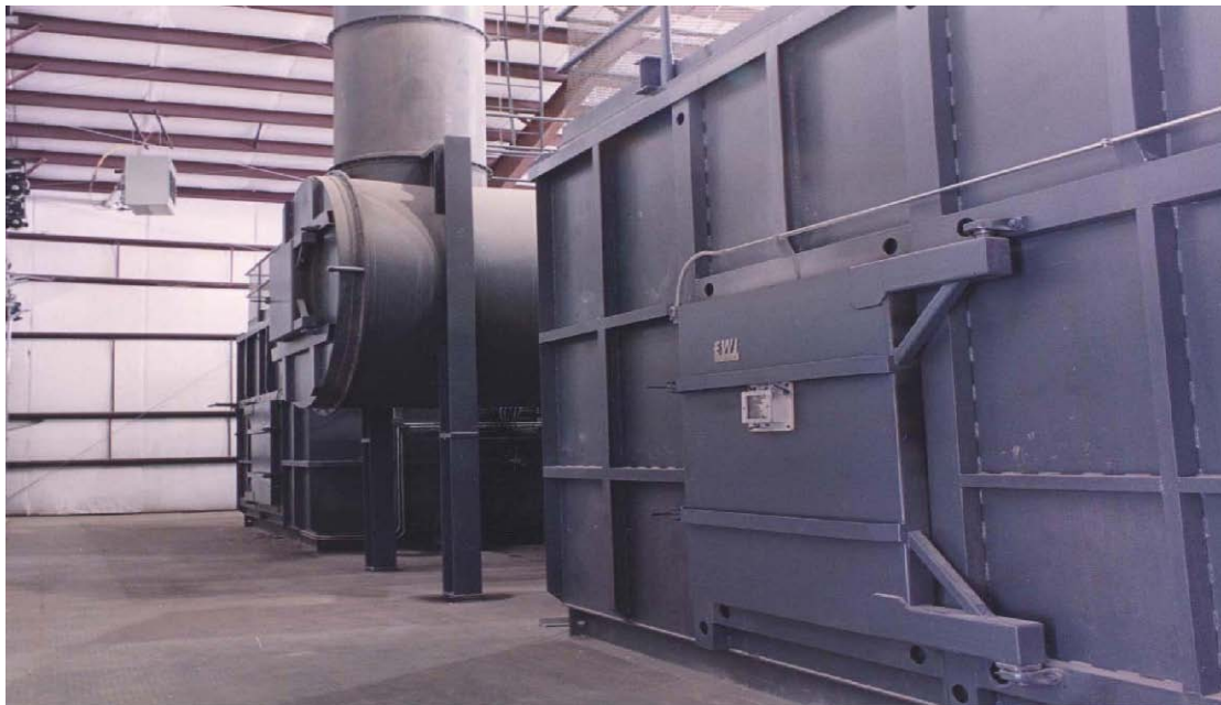
20 ton per day BOS located near Yellowstone National Park in Wyoming.
